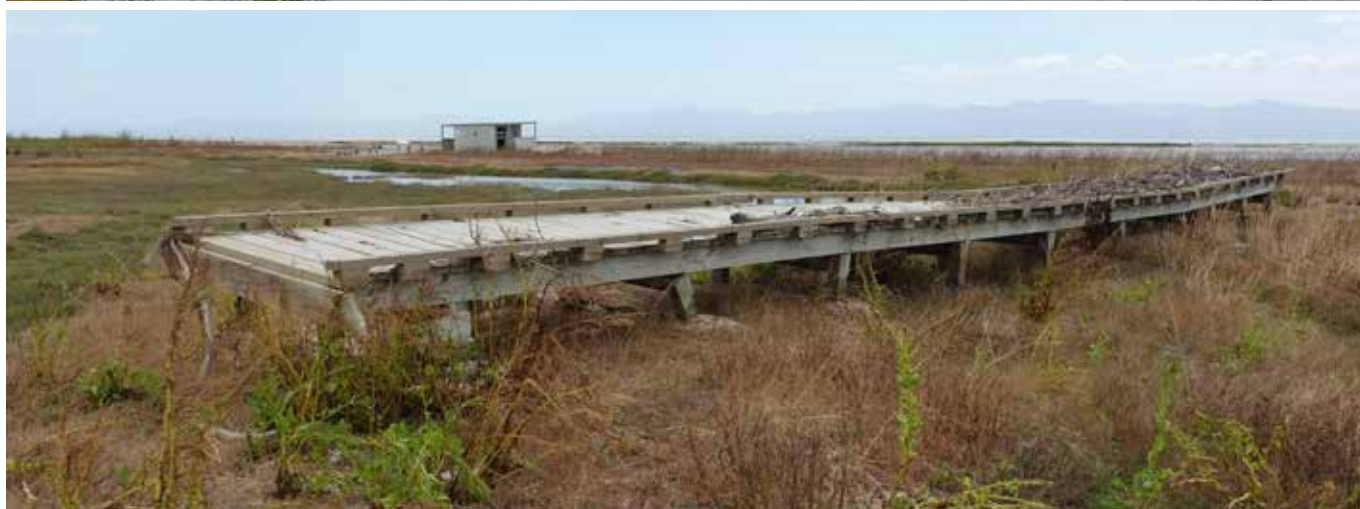
CUT OFF: (top) The storm swept away the boardwalk to the Godwit Hide. (below) the bridge ended up sitting firmly on its piles some 70m south. Photos / Chelsea Rails, Jim Eagles
